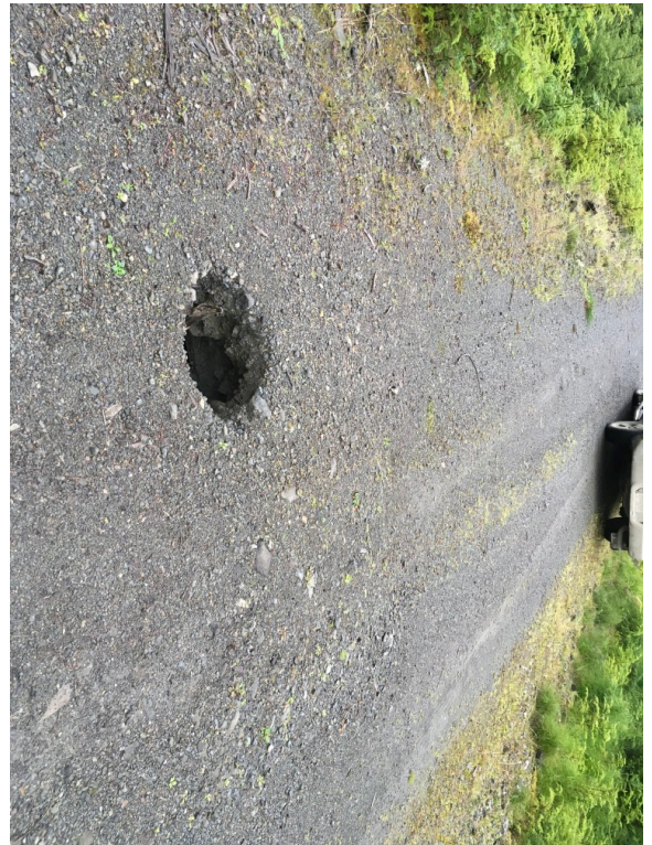
Hole in road
